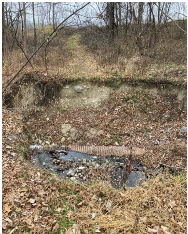
Damaged culvert on Dagmar Dale trail
